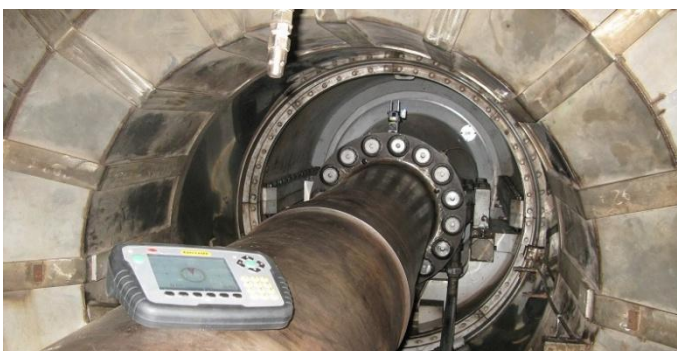
Turbine-Generator Shaft Alignment
