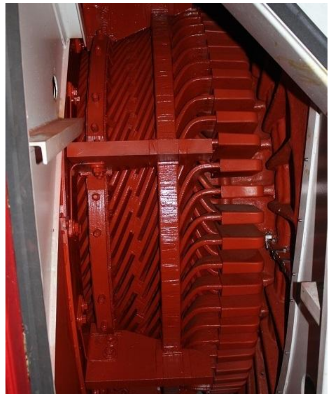
Part of the generator
